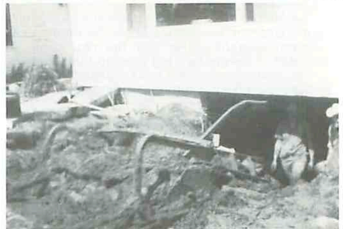
Cleaning out the basement of the Lutheran Parsonage after the flood caved in the basement wall.
